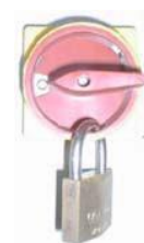
Main switch with padlock
